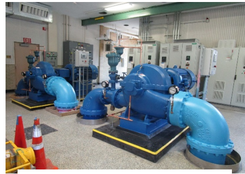
New Pumps Commonwealth Avenue
