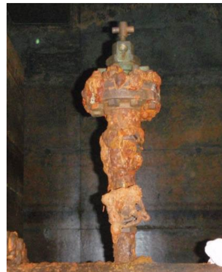
Corroded air valve at Shaft 9A
