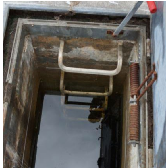
Flooded Shaft 7D valve chamber
