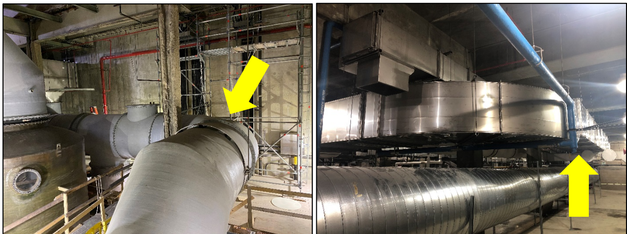
72-inch Odor Control Duct Requiring Sprinklers
